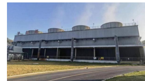
Circulating Cooling Water Tower
